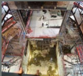
Installation of the modular stage floor has begun in the auditorium stage basement.
